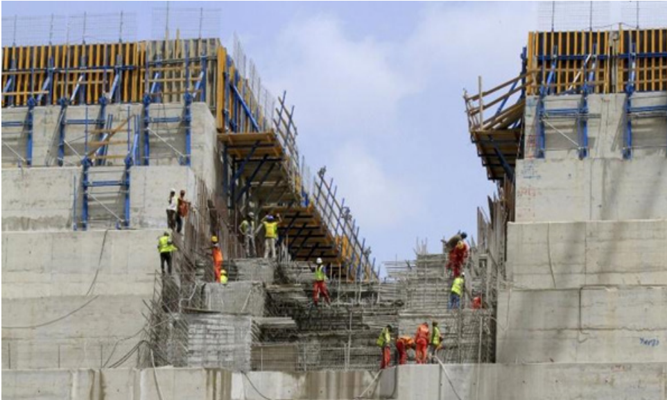
Figure 4.9. Workers are highly engaged in the construction of Ethiopian Grand Renaissance Dam
